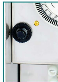
Magnetic circuit breaker on secondary to protect lighting system
